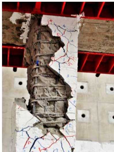
側位移比1.75%，混凝土嚴重崩落
